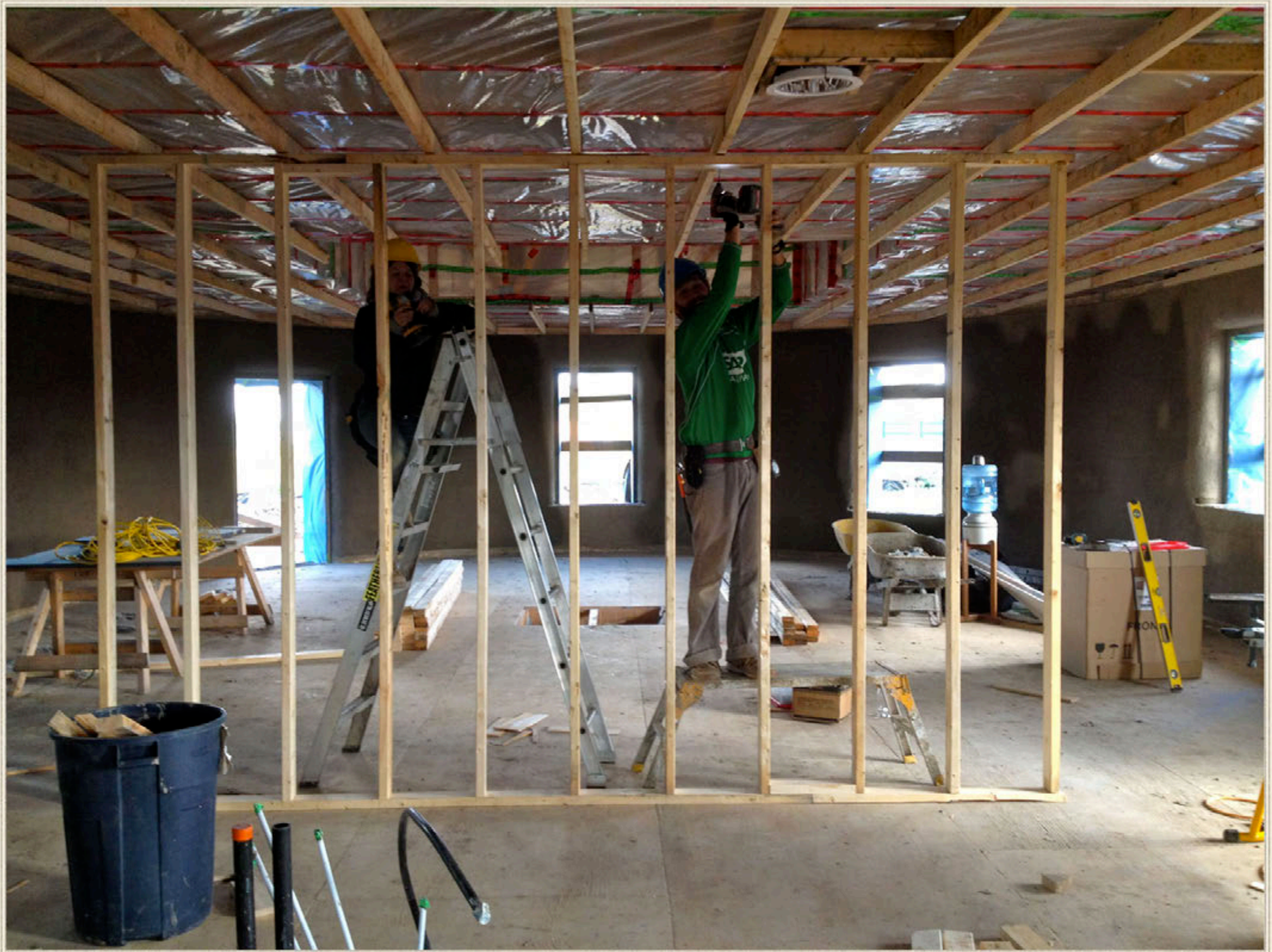
The ceiling is furred down to allow wiring to stay under the ceiling air barrier. Interior walls are conventional 2x4 framing.
