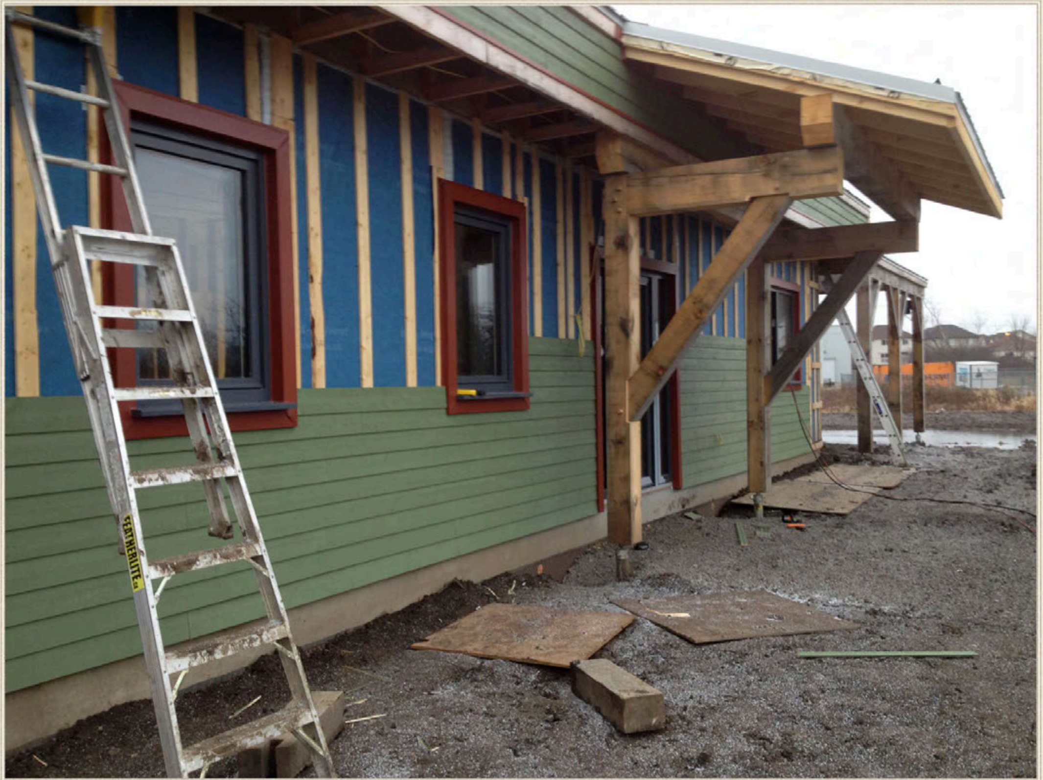
Horizontal wooden siding is used to clad the straight sections of the exterior walls.
