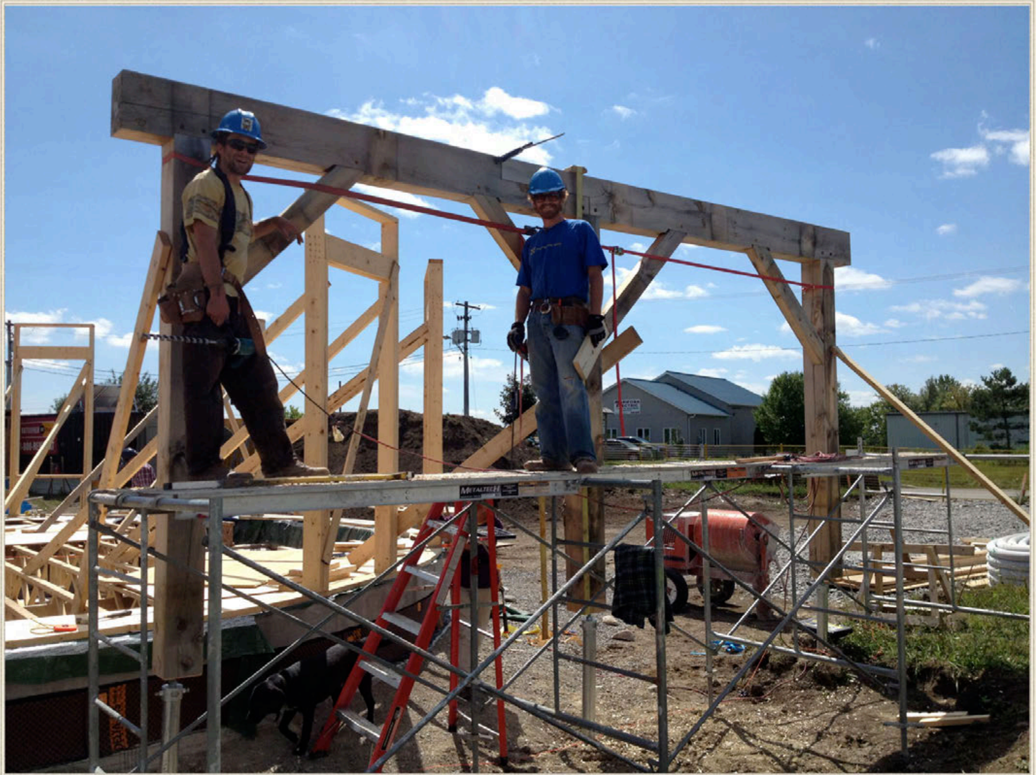
The timber frames are installed at all four corners of the building.
