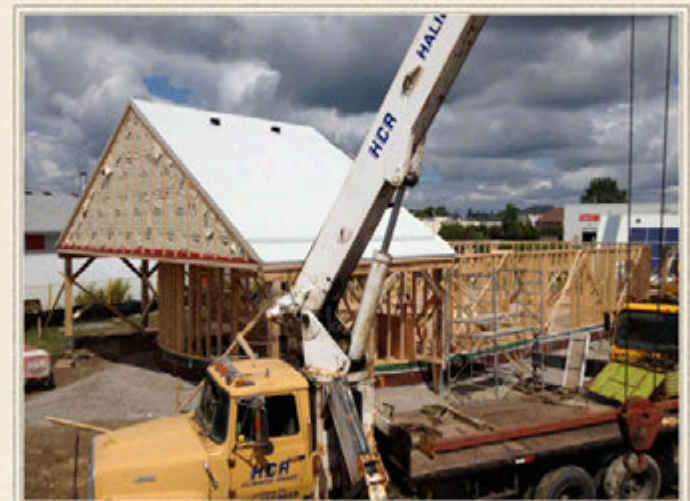
The roof sections are lifted onto the frame walls with a large crane in a single day.
