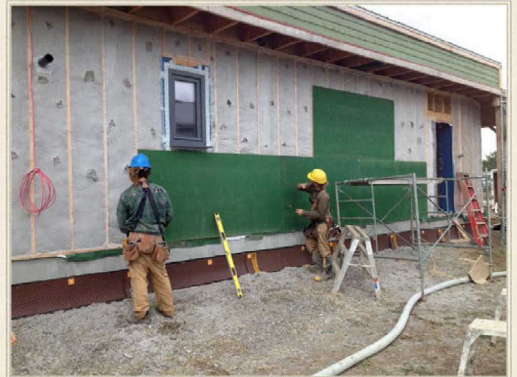
Cellulose is dense packed into the exterior wall cavities, and an insulated fiber board sheathing is applied.
