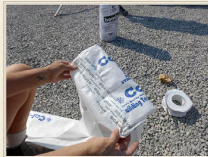
The first long tube of earthbag is prepared and installed onto the loader.
