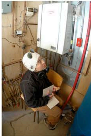
Boiler and header
