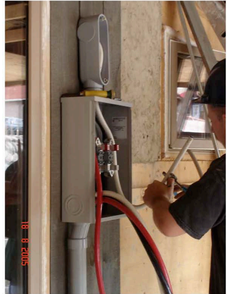
Grid tie meter base
