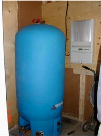
Solar hot water tank
