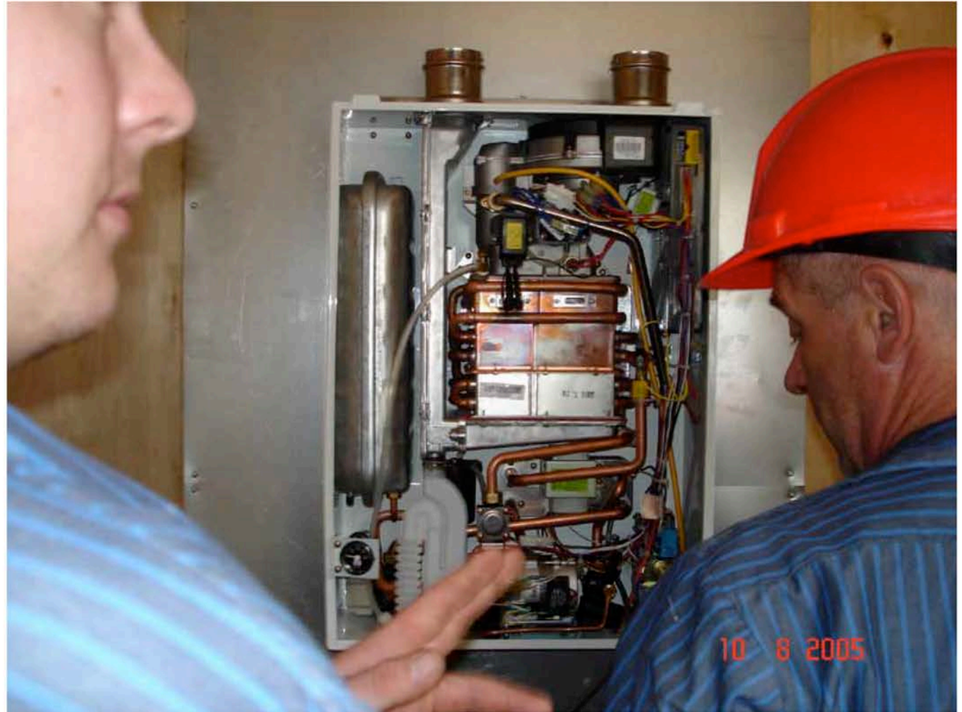
On demand boiler
